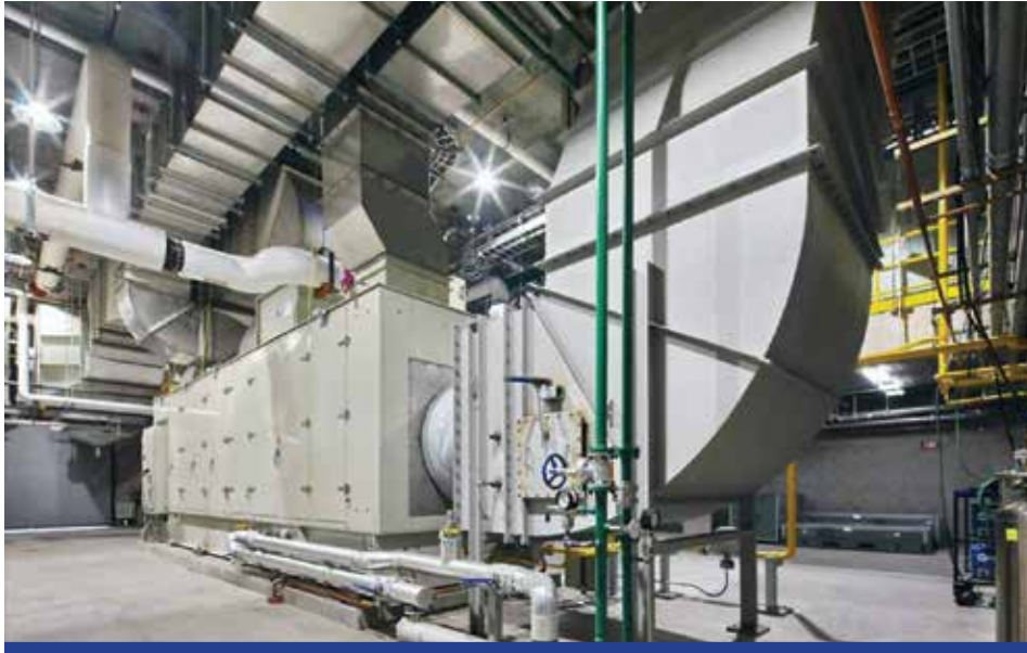
View from floor, showing Arizona State University's new turbine generator and associated industrial ductwork at the combined heat and power facility.
