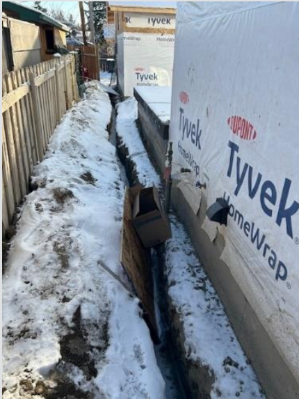
This site is not backfilled
