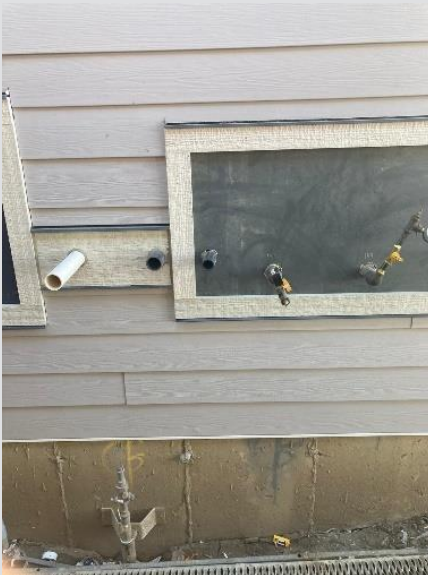
Insufficient clearance from appliance vent. Refer to Figure 5 for distances gas regulator must be from all appliance vents.
