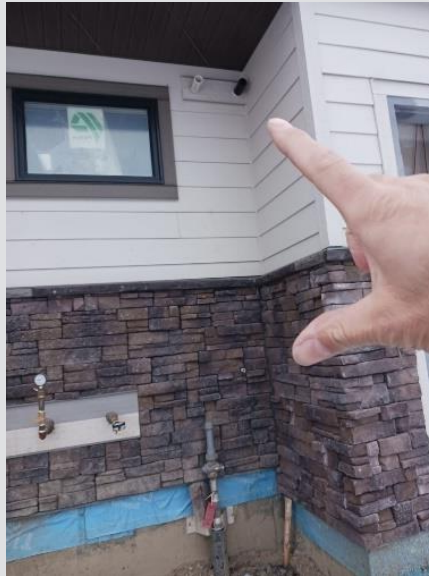
Insufficient clearance. There cannot be venting within 15' of the top of the regulator. (Refer to Figure 5)
