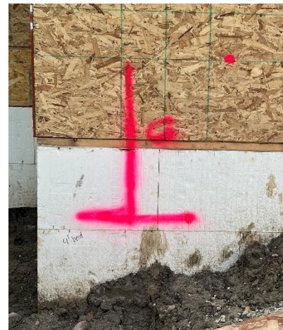
Figure 7: Gas riser location marking
