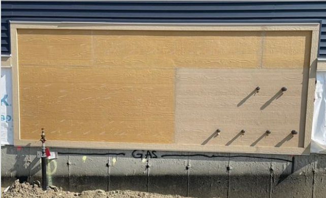
Houselines are too far away from the service riser. The first houseline should be between 20" and 30" from the service riser.
