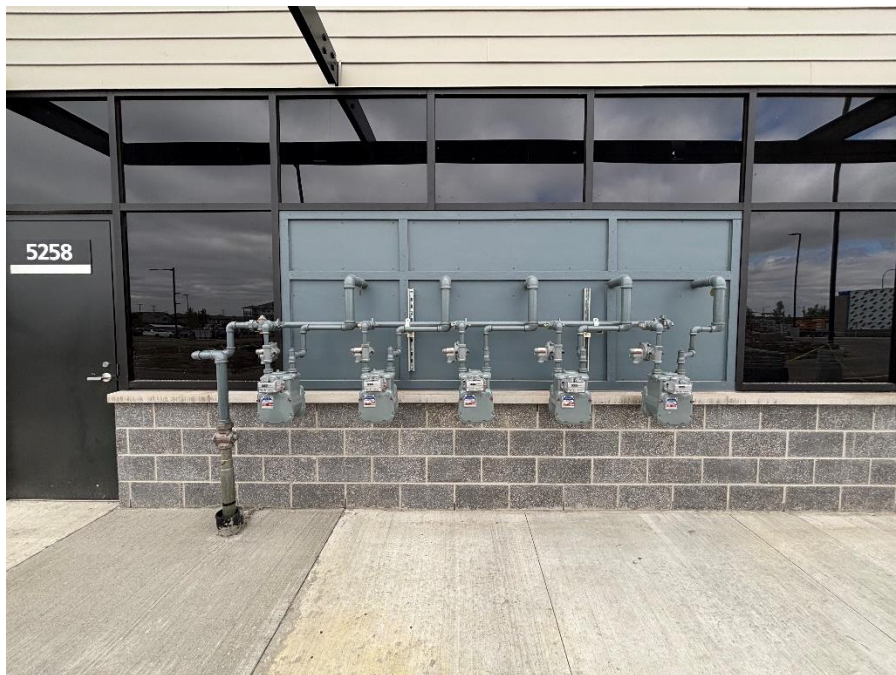
Figure 17: A good example of a commercial backing-board set; the customer installed a backing board (grey) so we could mount meters
