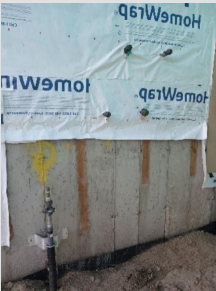
There is no backing board and the houselines are staggered. They should be in line with each other, up and down, and there should be a backing board
