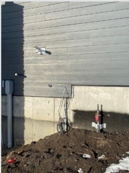
The houseline is too far away and on the left side of service. It must be within 16 – 24" to the right of the riser.
