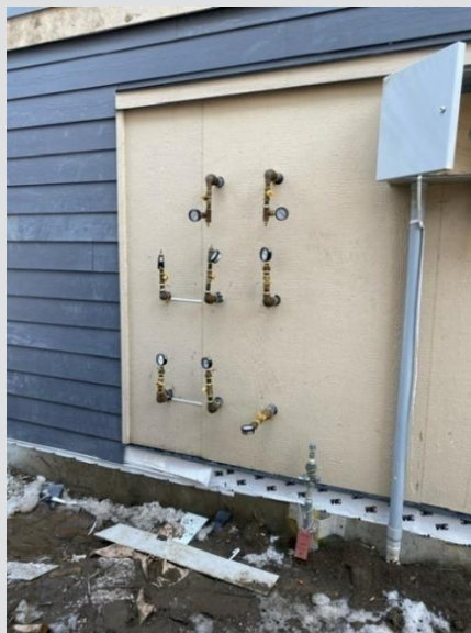
A maximum of 2 rows is allowed for stacked meters to allow for future access for maintenance.
