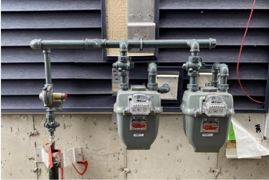
Figure 11: Residential Two-Meter Manifold with an alternate style backing board (Figure 12)
