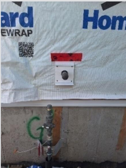
The houseline is too close to service. It must be 16 – 24" to the right.
