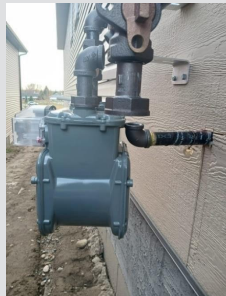
The houseline is too long. Houselines must protrude 3 – 4.5" from the final wall.
