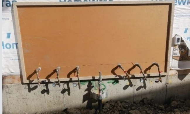
Houselines must only come out on one side of the riser. The riser cannot be in the middle.
