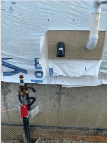
Appliance venting is too close to service (must be 1 m), and in the spot the meter needs to be placed
